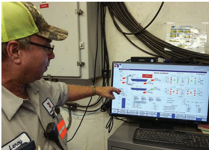
Division Environmental Manager Leroy Woody discusses aspects of the SCADA system used to balance and manage wastewater treatment operations. | Courtesy of American Proteins
